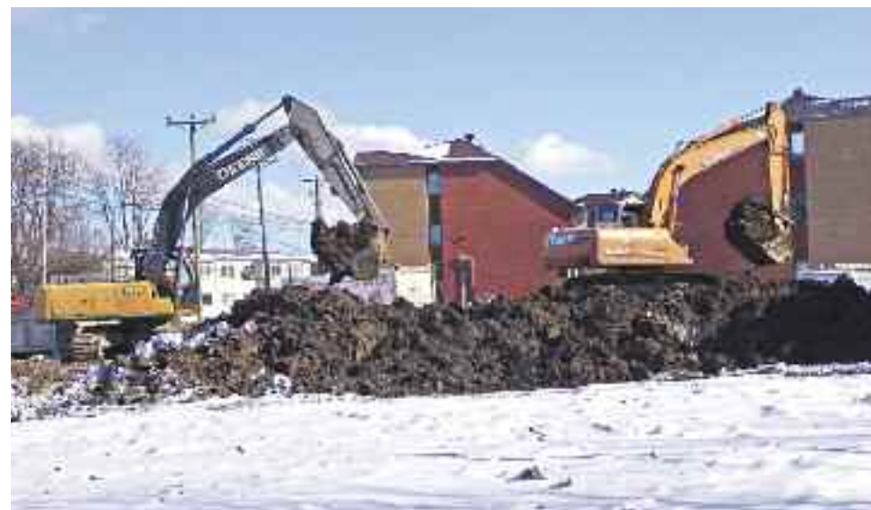
Crews move earth near the Côte St. Luc Aquatic and Community Centre. Starting in April, crews will begin building an apartment tower here on Parkhaven Ave.
